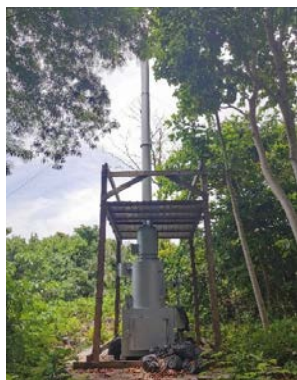
Figure 47. SMOKELESS INCINERATOR INSTALLED PRIVATELY AT THE REEF DIVE RESORT
